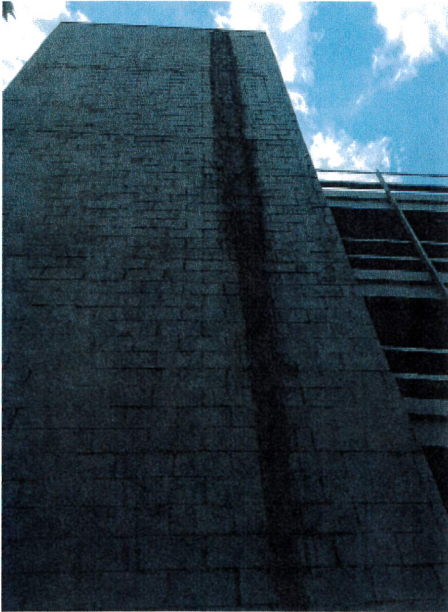
Picture #2. Stairwell CMU cracks
