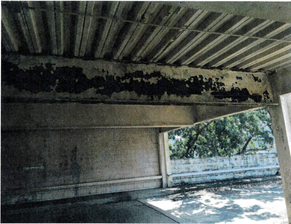
Picture #8. Rust on steel beam
