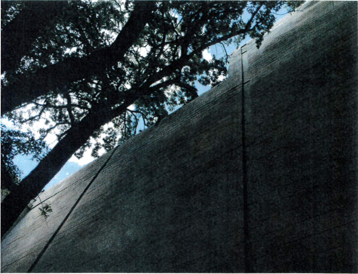
Picture #5. Cracking in parapet of CMU end wall.
