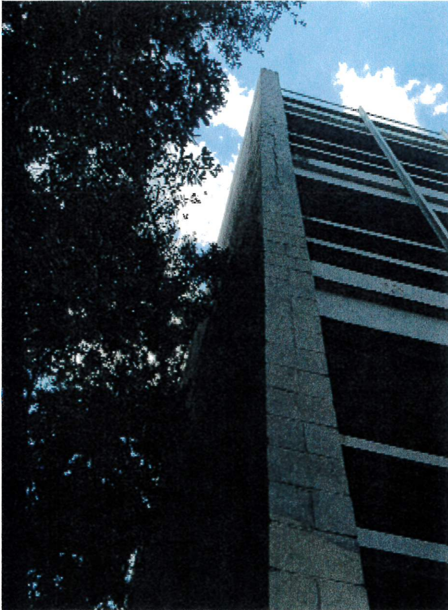
Picture #4. Cracking in CMU end wall
