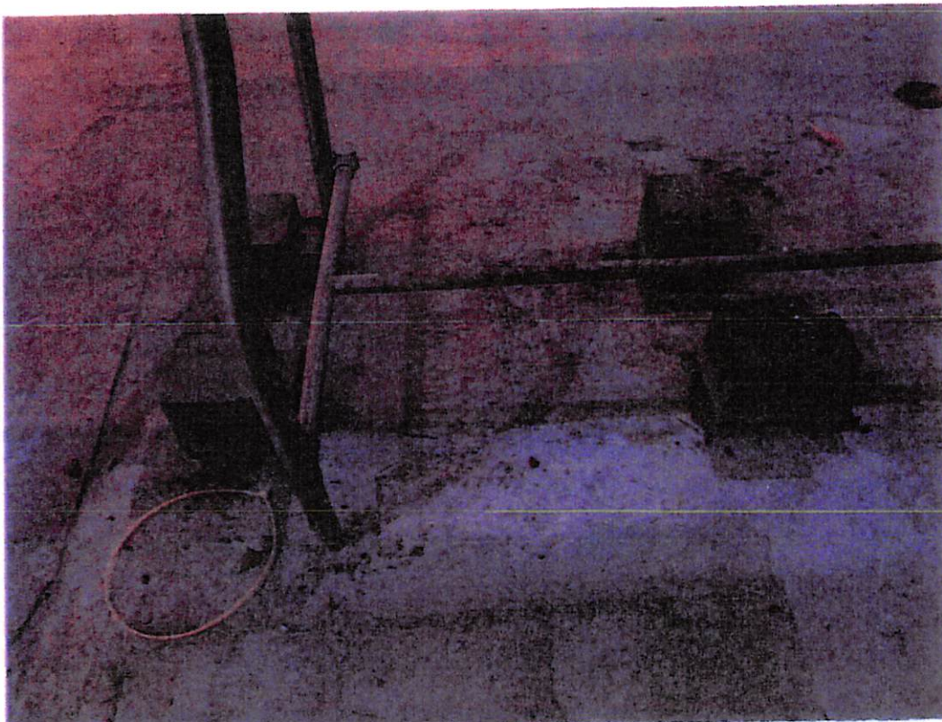
Floor Under Serving Line in Kitchen
