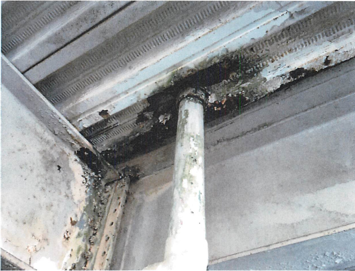
Picture #10. Rust on steel beam and corroded steel deck.
