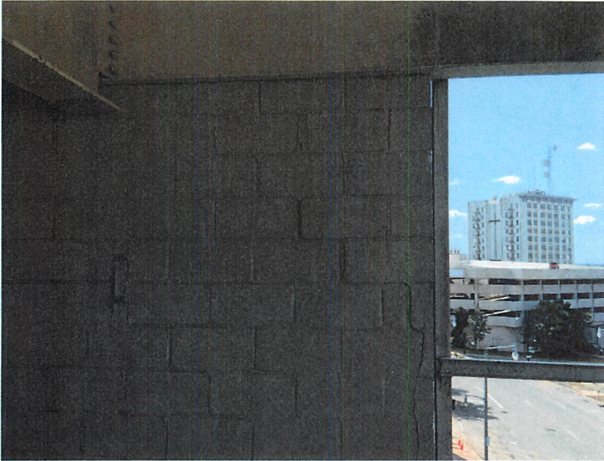
Picture #3. Stairwell/elevator shaft CMU cracks
