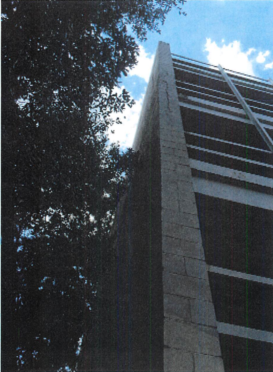
Picture #4. Cracking in CMU end wall
