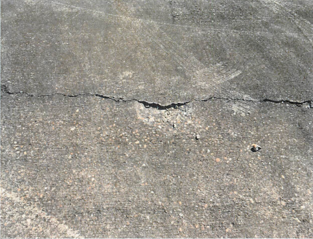
Picture #12. Crack in top level over a beam line.
