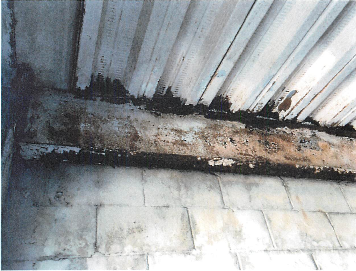
Picture #9. Rust on steel beam
