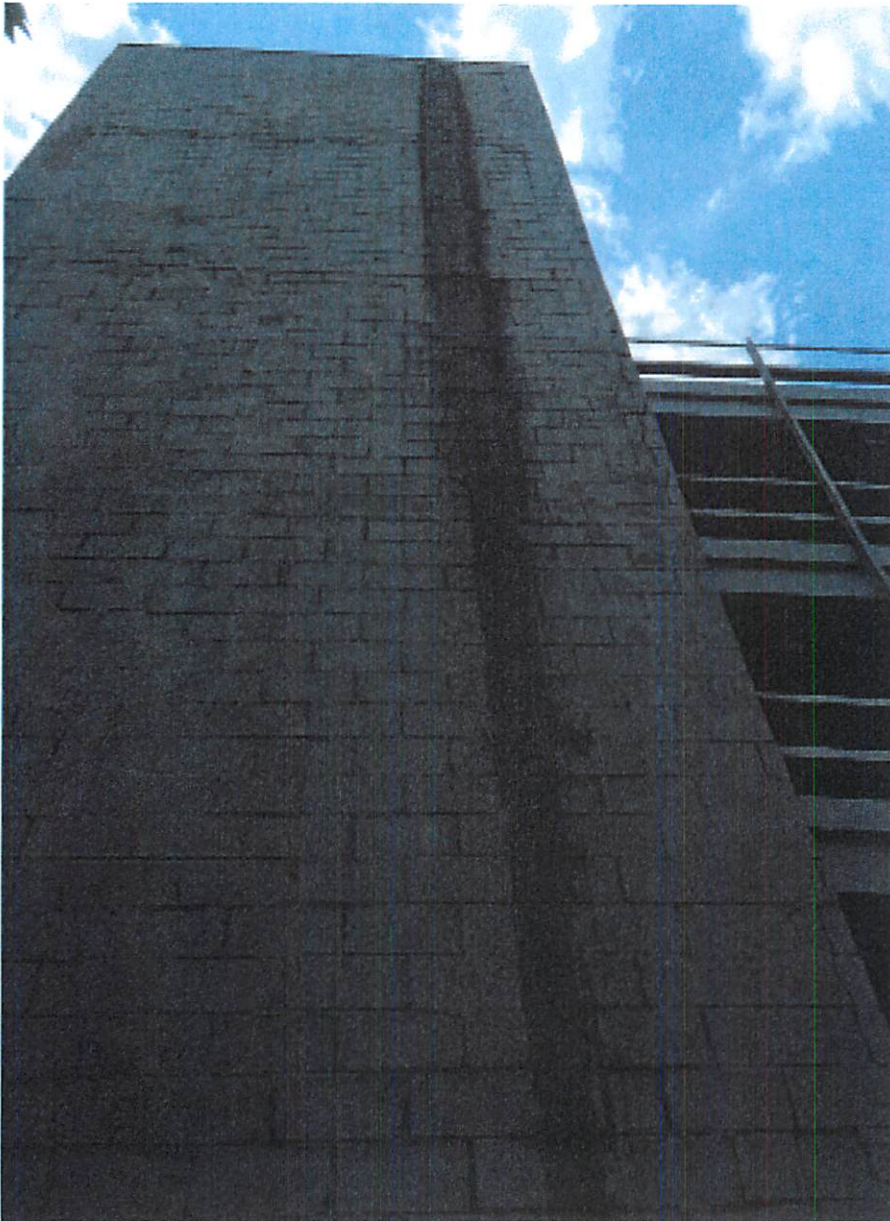
Picture #2. Stairwell CMU cracks
