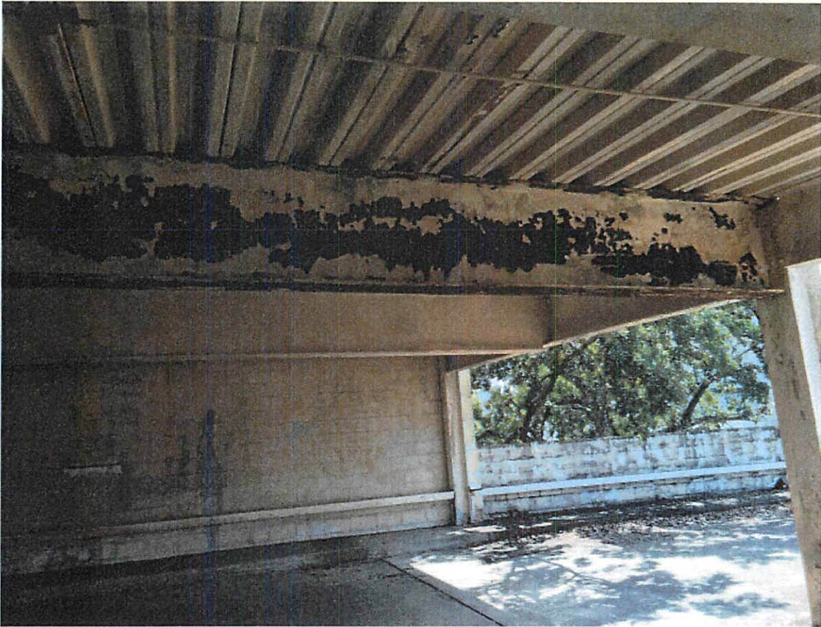
Picture #8. Rust on steel beam
