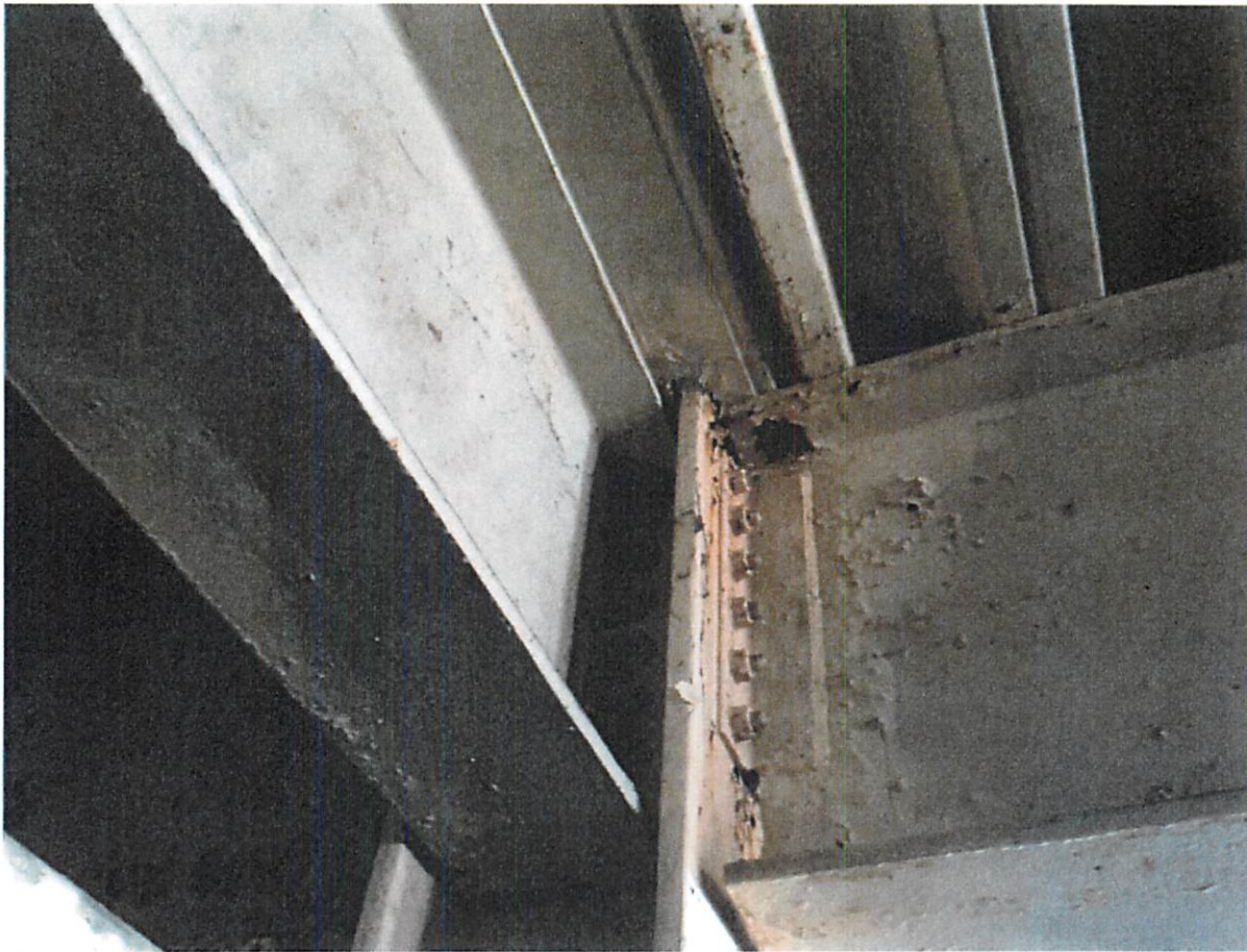
Picture #7. Rust on steel beam
