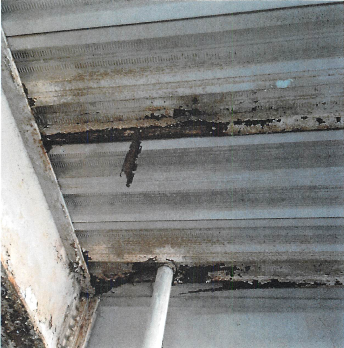
Picture #11. Rusty deck and beam
