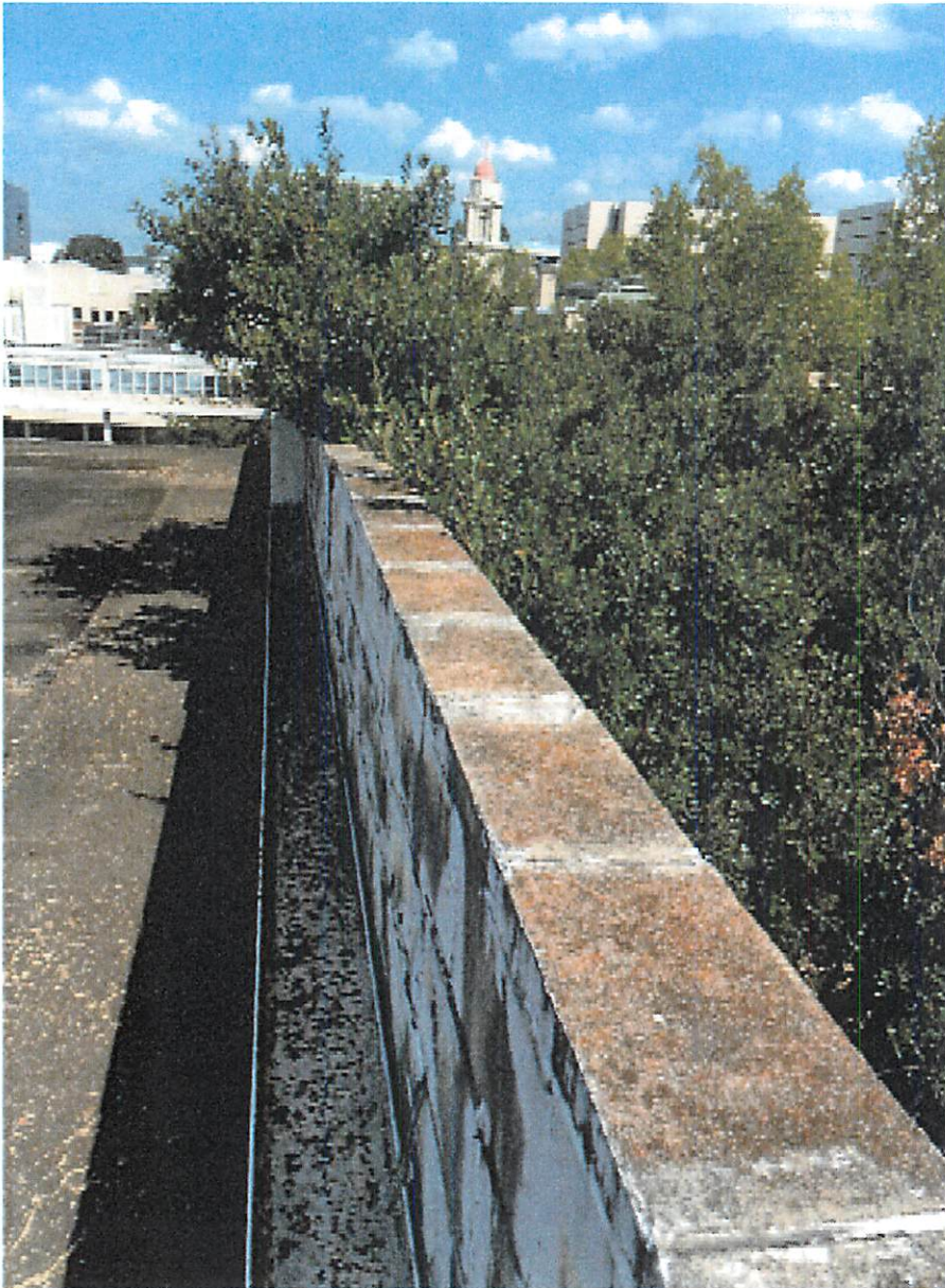
Picture #6. Overgrown vegetation
